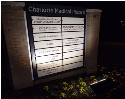
Solar Flood Light - 20W, 2000 Lumens Charlotte Medical Plaza, NC
